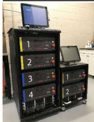
Figure 15: DDC battery station
